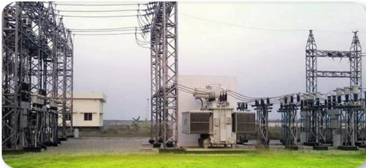
Newly Constructed 33/11KV, 2x8 MVA Substation at BEZA, Mongla.
