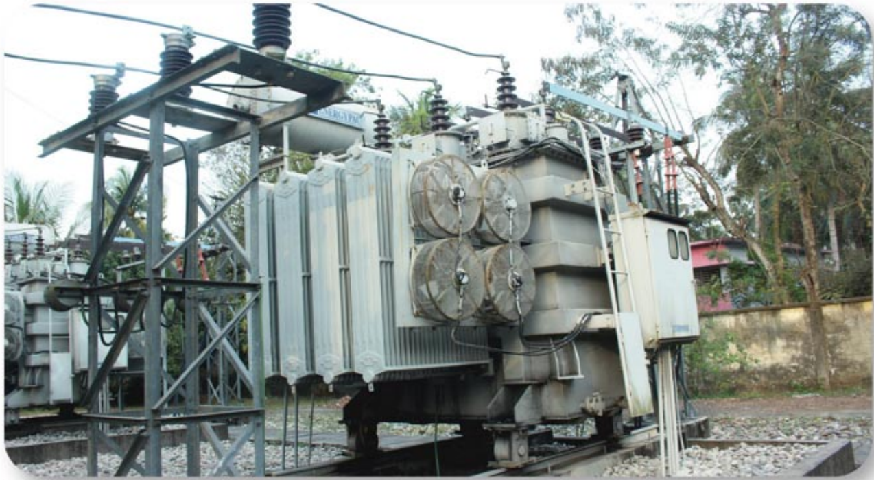
33/11 kV Substation, WZPDCL
