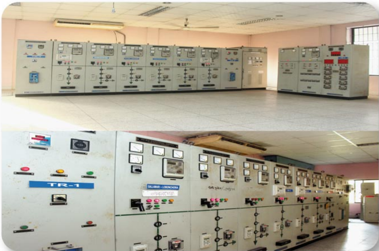
Control Room of Pather Bazar 33/11 kV Substation
